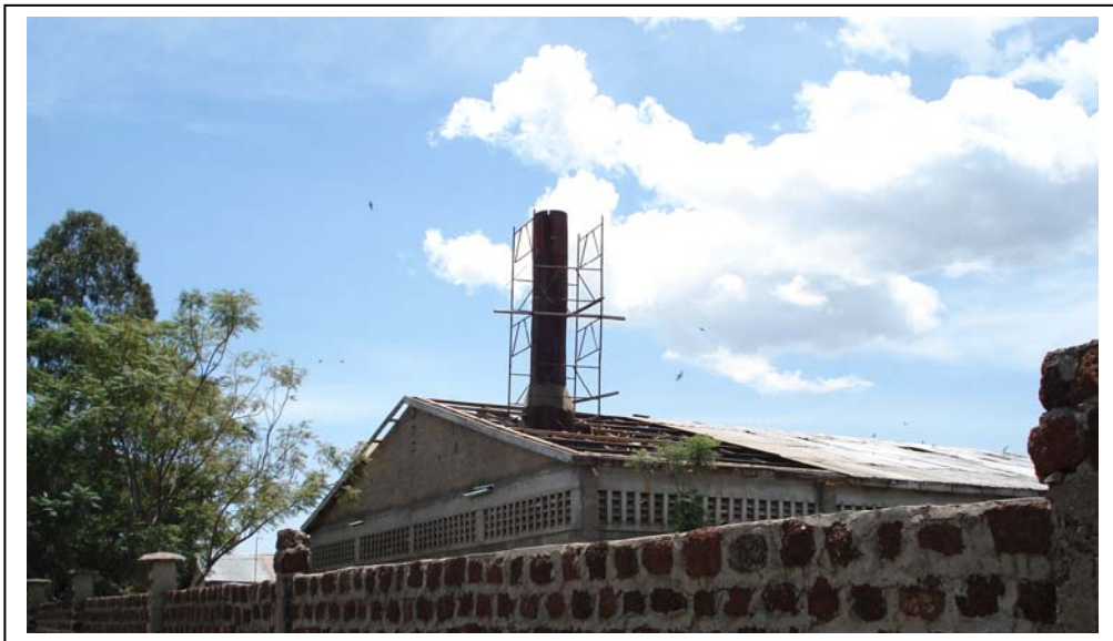
Figure 3: Part of the corroded and blown out roof of Bondo Fish meal ltd
